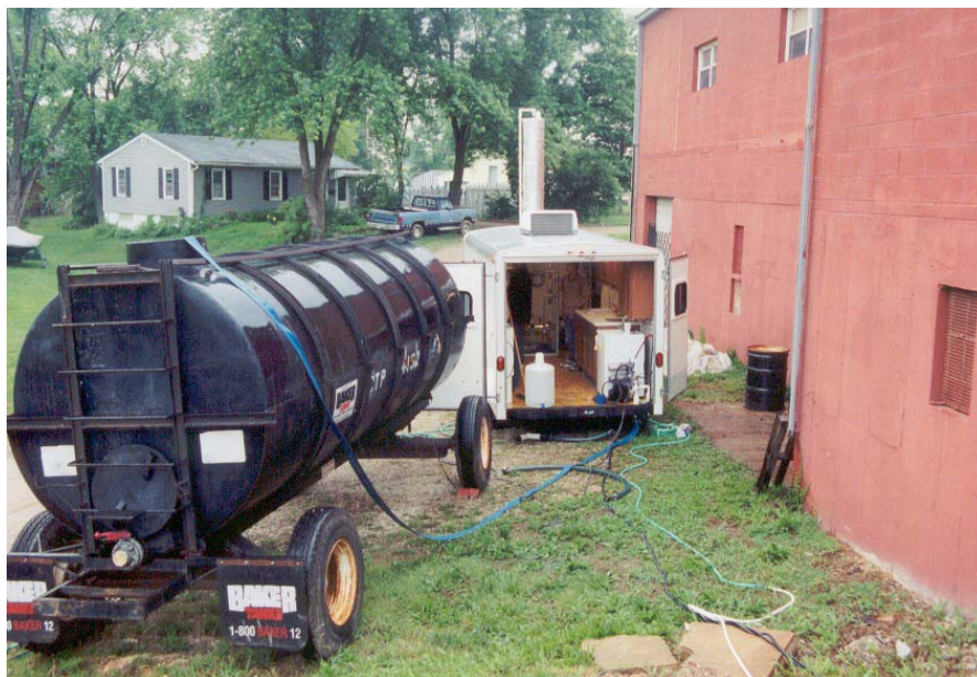
Figure I -6. Mobile water treatment plant on site.
