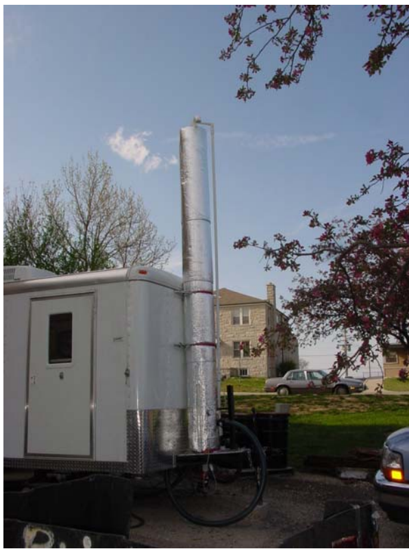
Figure II-5. Packed tower mounted on trailer.
